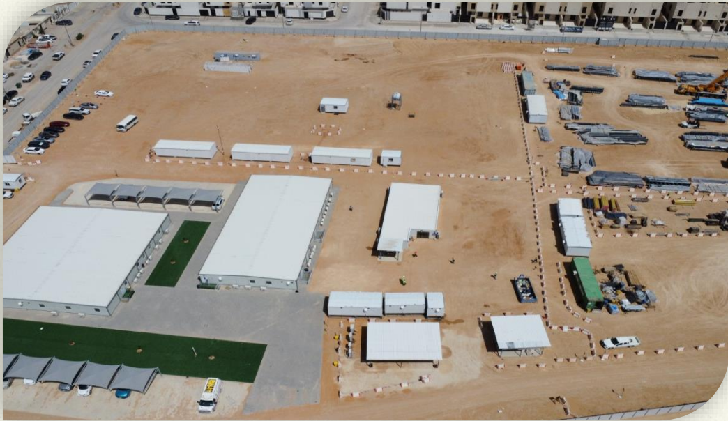
Supported Execution of a turnkey contract for setting up of a Data Centre Project in Riyadh, Kingdom of Saudi Arabia.
