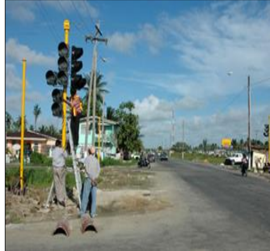
Supply and installation of traffic signaling system under Exim Bank's GOI-supported Line of Credit to the Government of Guyana .
